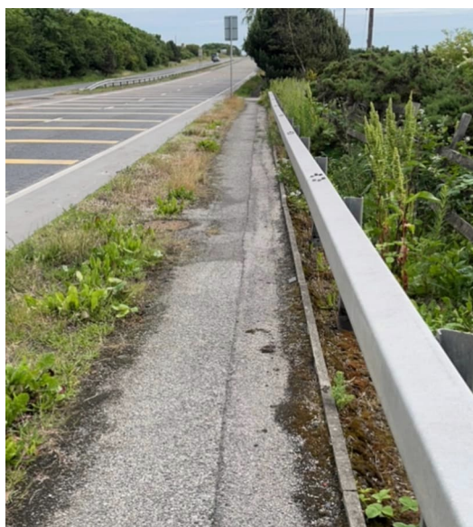
Figure 1 Existing Footway Condition - VRS
