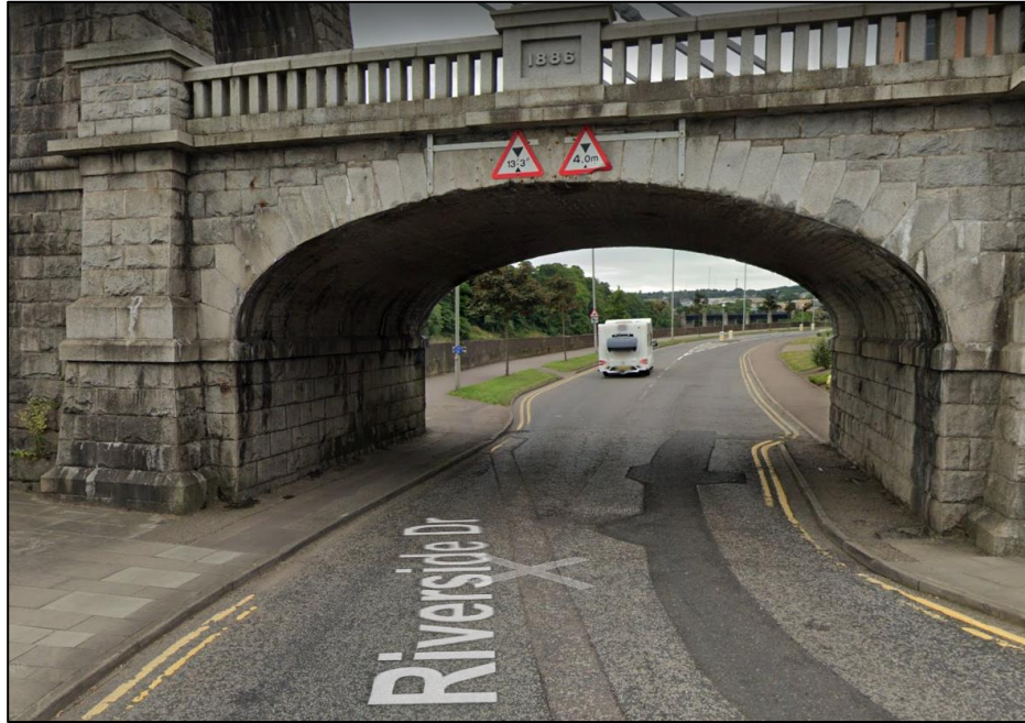
Figure 7. Narrow Footways Under Wellington Suspension Bridge (Source: © 2023 Google)
