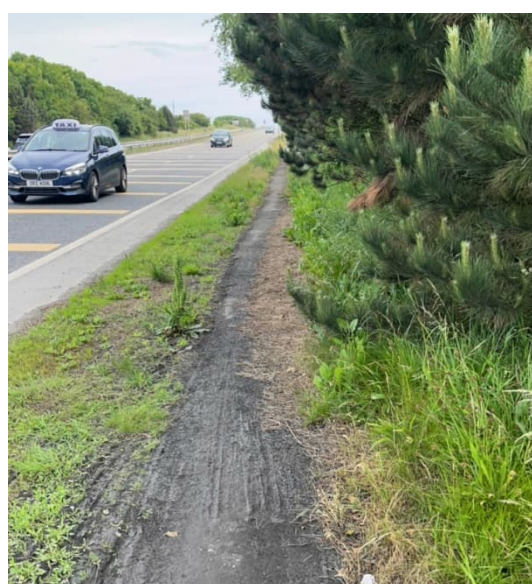
Figure 2 Existing Footway Condition - Overgrown Vegetation
